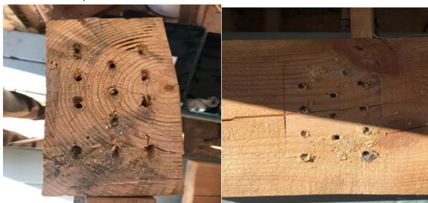
FIGURE 9 The nature of beam joint destruction:( a) secondary beam and (b) main beam
